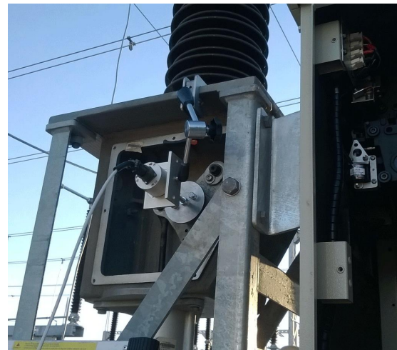
Figure 2: Digital rotary transducer mounted on ABB LTB 245 kV SF6 circuit breaker
