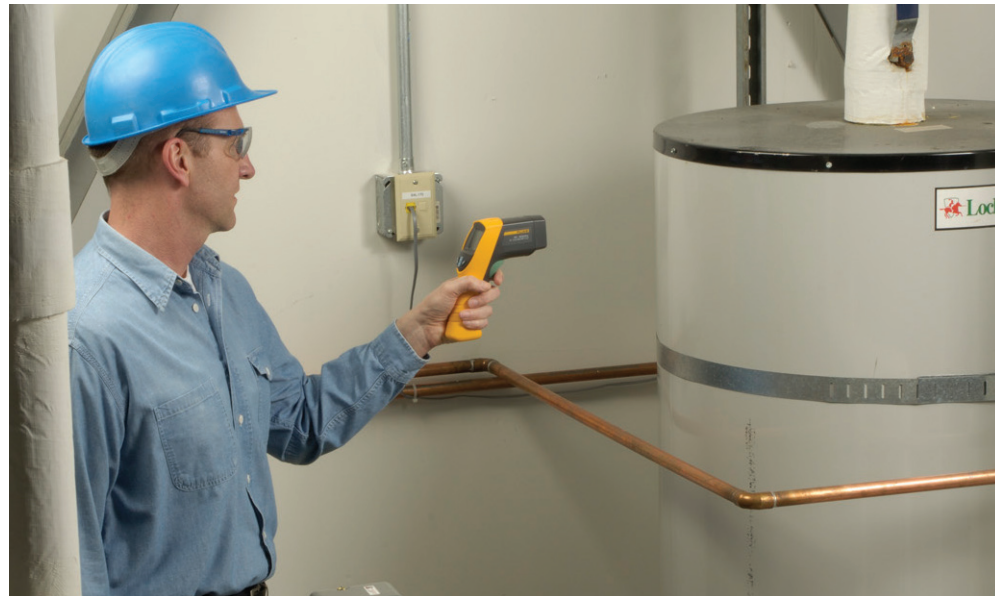
A quick infrared survey can check for leaks and uneven temperatures in both the heater and pipes.
