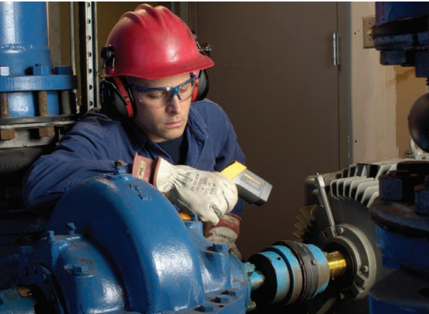
Measuring chiller pump motor bearing and case temperature.
