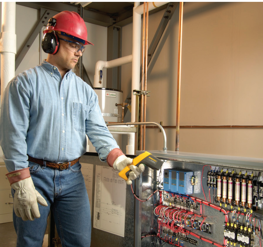
Measuring temperature of fuses and electrical connections.
